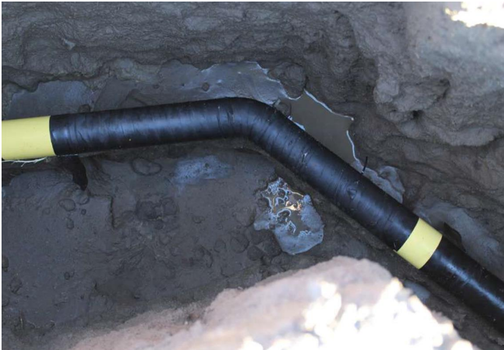
Figure 1 A confirmed 1.5d, 45 deg. bend in the pipeline.
